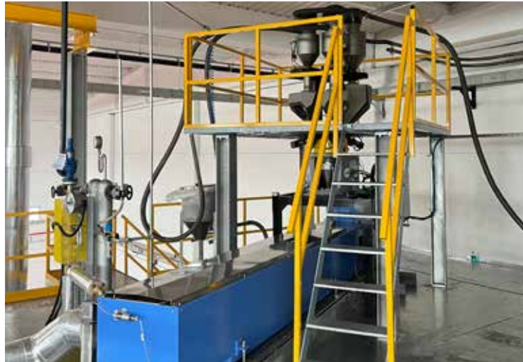
Extruder with dosing system
